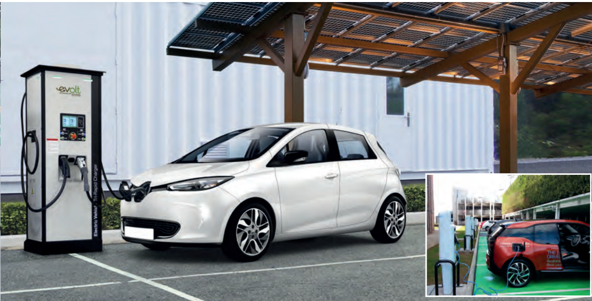
Far left: The UK government recently awarded US$50m to Go Ultra Low Cities to encourage PEV uptake Left and inset: By 2020, there will be more charging points than gas stations
