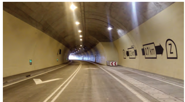
The newly built D3 required planners to follow EU directives on tunnel safety requirements
